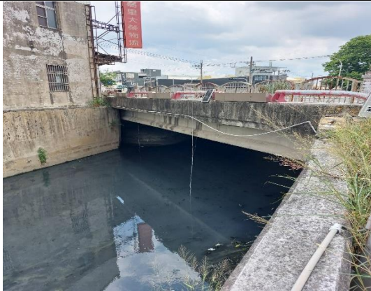
Mobile Sensor Installation Completed
